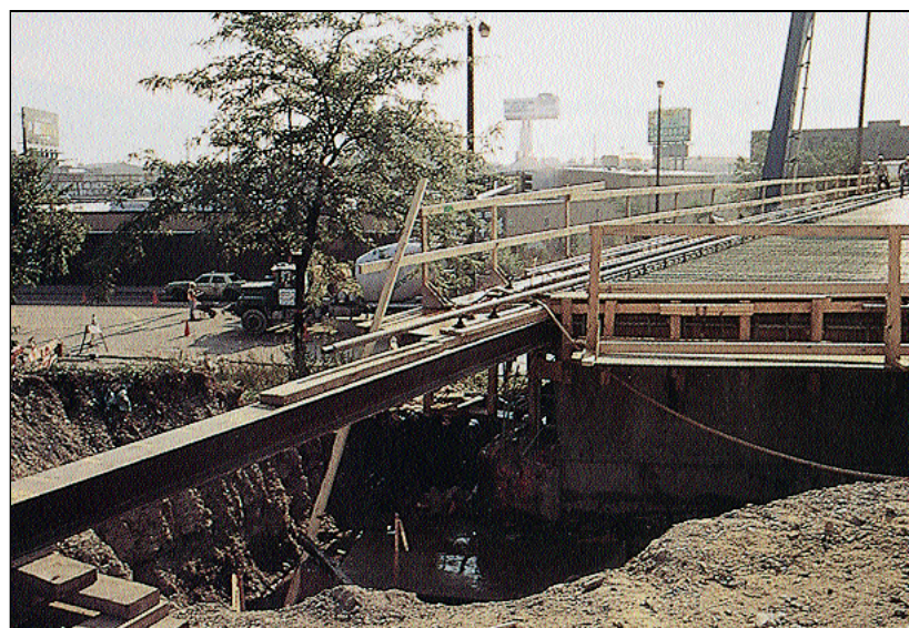
Figure 2. Extend the screed rail beyond the limits of the concrete placement to ensure grade at end bulkheads and to operate the paving rollers, screed pan, and drag to the end of the concrete placement. On this job, the contractor provided temporary blocking to support the screed rail beyond the concrete placement.
