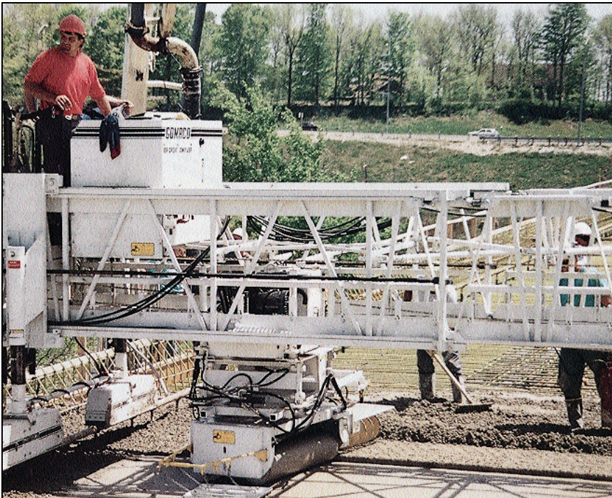
Screed rail used to set deck slab grade for paving machines can be set on the exterior overhang form or on the exterior girder. Placing the screed rail on the girder requires hand placing and finishing of side strips.
