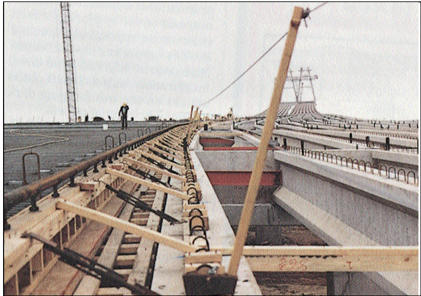
Figure 3. Use a 2x4 stud wall to support screed rails on the exterior formed overhang. Brace the wall every 2 to 3 feet and drill holes every 24 to 32 inches to insert threaded rod for screed chairs.
